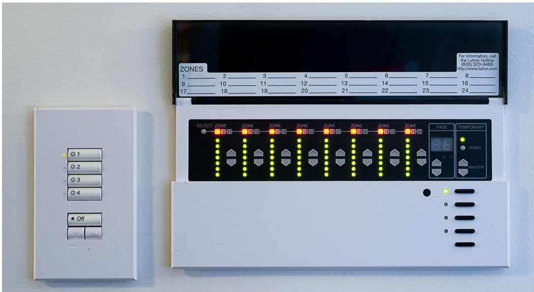
Figure 1.1: A lighting control panel found in a modern building, allowing control of 24 dimmable zones. (Lutron Grafik Eye 4000 [23] system.)
